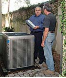
Tommy Castellano of Castellano Air Conditioning and Heating Inc. discusses his company's installation of a York condensing unit with a homeowner.
